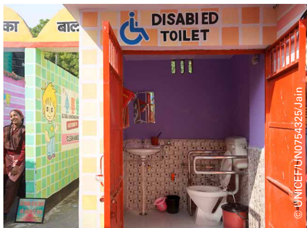
An accessible toilet at Uchhattar Prathamik School in Uttar Pradesh, India.
