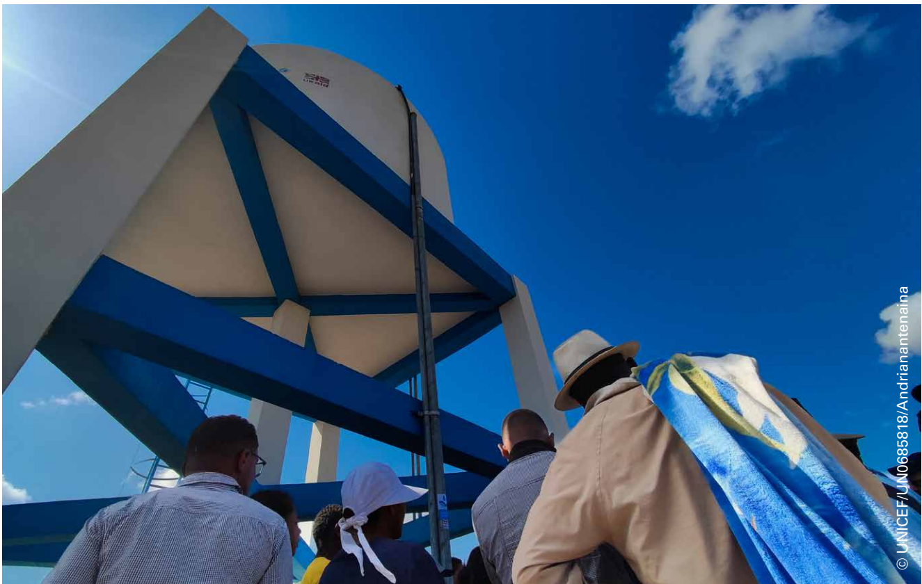
The water tank of a new solar-powered water system in the community of Androimpano, southern Madagascar, constructed by UNICEF with the support of the Government of the United Kingdom.
