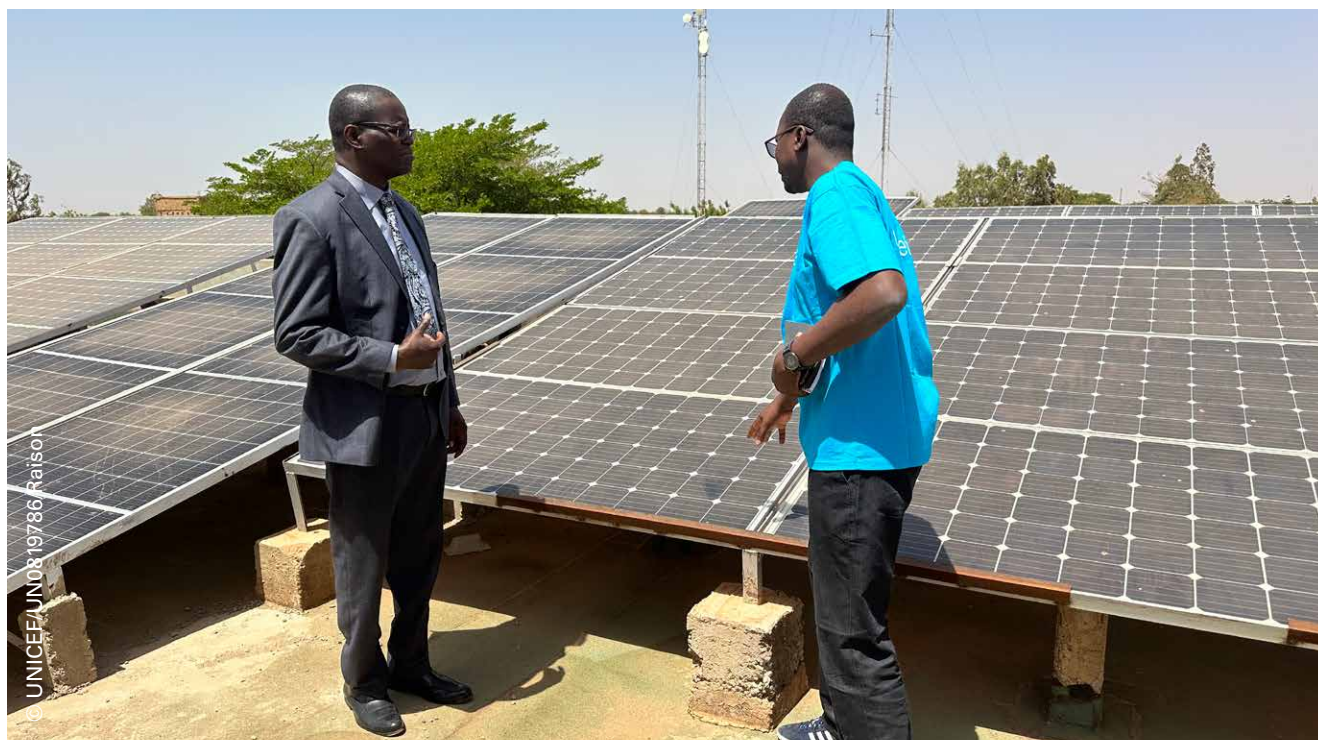
UNICEF staff inspecting solar panels on the roof of the UNICEF office in Mopti, Mali.
