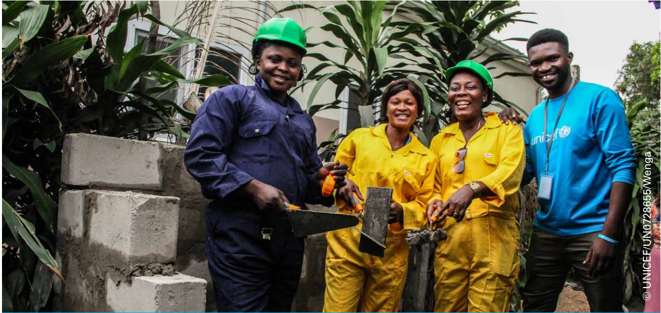
Women in the commune of N'Sele in Kinshasa, Democratic Republic of Congo in a training programme supported by UNICEF and the Bill & Melinda Gates Foundation on toilet construction.
